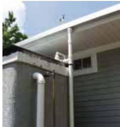
Cistern collects rain for nonpotable uses.
